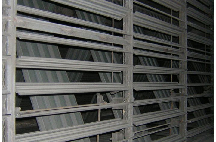
Air dampers like these need to be checked as part of a freeze rounds routine. BMS data isn't always accurate.
