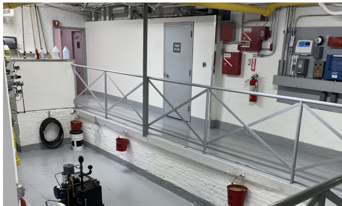
An Adams & Company facility demonstrating exemplary sanitary and safety protocol compliance
